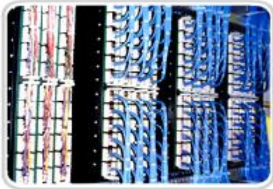
UTP patch panels in a rack
